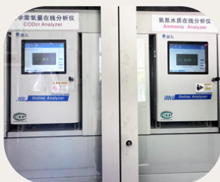
Wastewater monitoring devices in Shanghai, China
