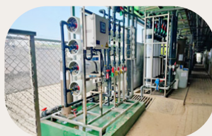
Reverse osmosis treatment on wastewater
